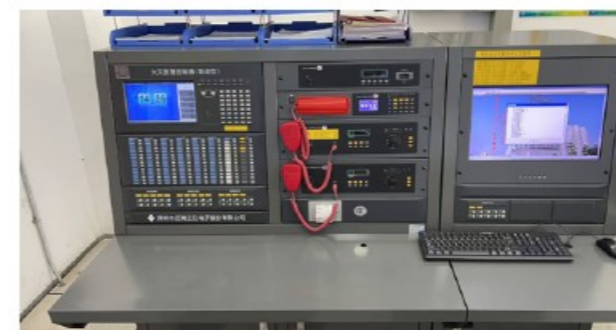
Fire Alarm Controller
