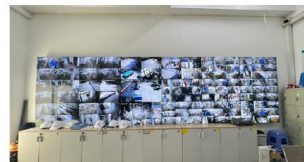
Smart Monitoring Platform
